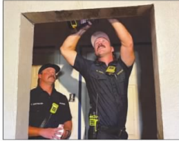
The Tyler Fire Department went door-to-door, changing batteries and installing new fire alarms in homes surrounding Caldwell Zoo and Wolder Park to enhance fire safety in the community. (Contributed Photo/City of Tyler)
